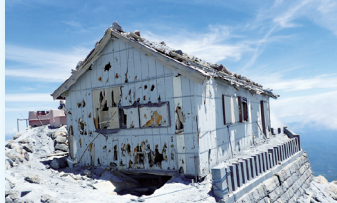
▲ Ontakesan: Building damaged by rocks and debris (June 10, 2015) <Photo by Ontakesan Joint Observation Team>
