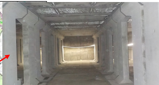
都雨水貯留槽 貯留量: 2,600m 3
