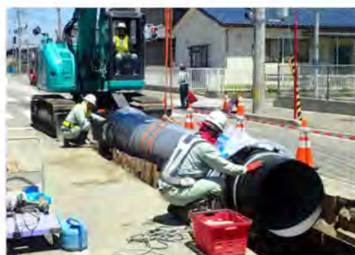
Installation of ductile cast iron pipe (earthquake-resistant joint (NS type), pipe diameter 700 mm)
