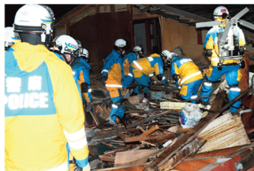
Nighttime activities at the site of a collapsed house (Suzu City) Source: National Police Agency
