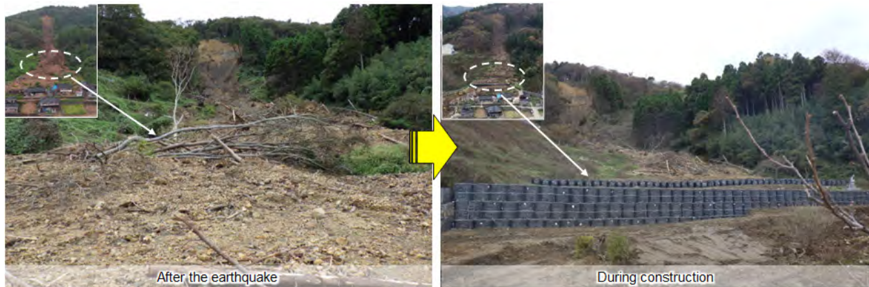
Forest under construction as part of a disaster restoration project (Oya-cho, Suzu City, Ishikawa Prefecture)
