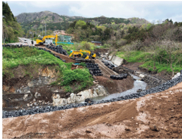
Construction of landslide prevention work under delegated authority (Wajima City, Ishikawa Prefecture)
