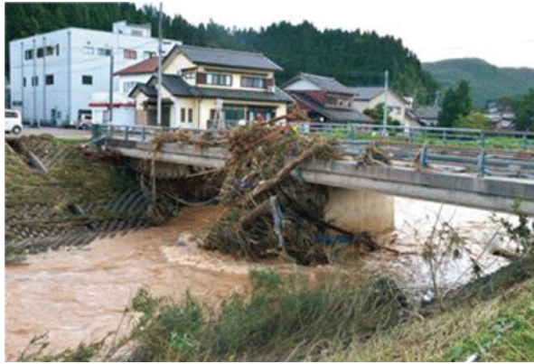
Noto Town Yanagida Noda Bridge area Source: Ishikawa Prefecture website
