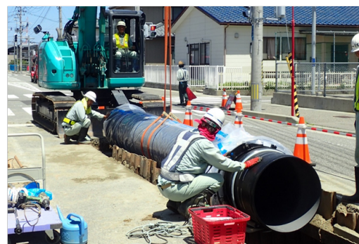
Installation of ductile cast iron pipe (earthquake-resistant joint (NS type), pipe diameter 700 mm)
