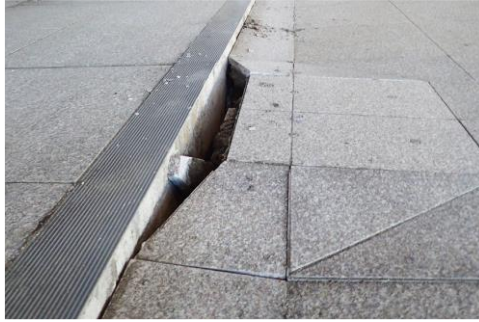
Cracks in the road surface (Soma City, Fukushima Prefecture)
