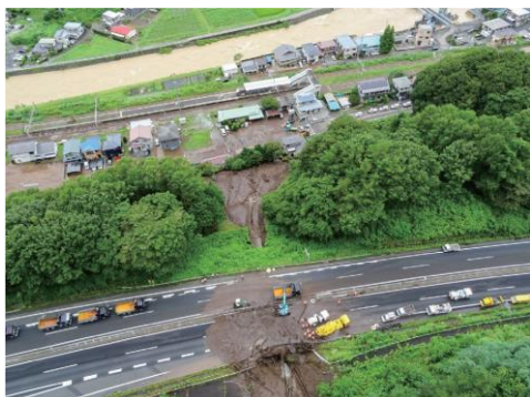
Slope failure damage in Okaya City, Nagano Prefecture (Source: Cabinet Office data)
