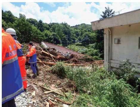
Slope failure damage in Unzen City, Nagasaki Prefecture (Source: Cabinet Office data)
