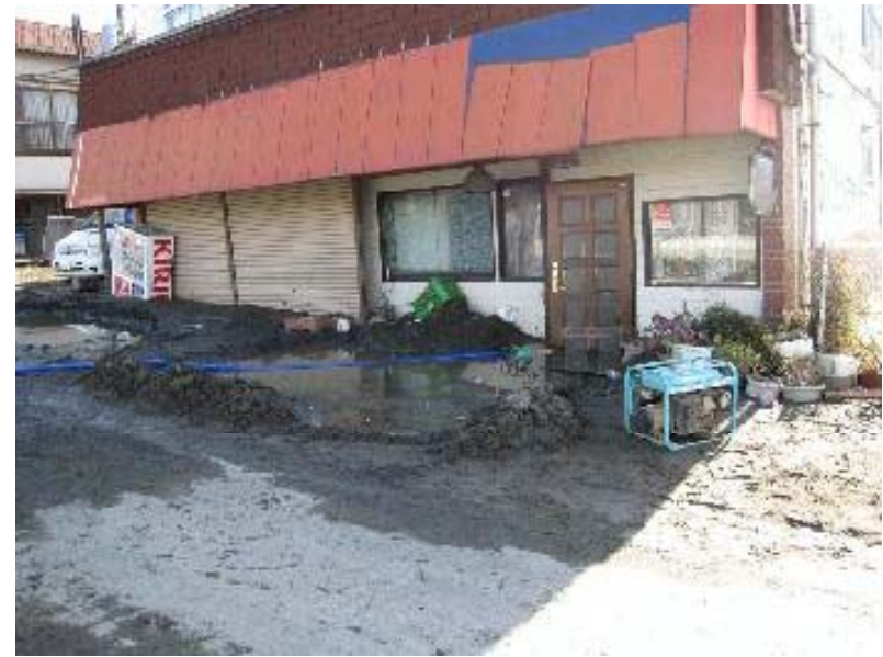
Buildings damaged by liquefaction (Abiko City, Chiba Pref.) (Photo: Abiko City Homepage)
