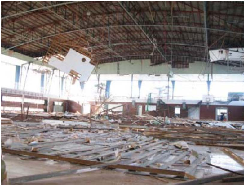
Ceilings and lights fallen in school gymnasium (Hitachi City, Ibaragi Pref.) (Photo: National Institute for Land and Infrastructure Management, Building Research Institute)
