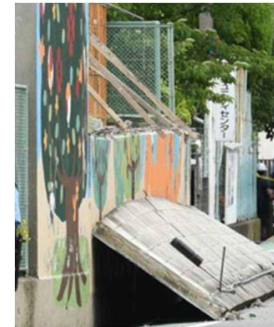
Concrete block wall of a swimming pool that collapsed due to the earthquake (Jyuei Elementary School, Takatsuki City, Osaka Prefecture)
