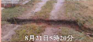
堤防天端の敷砂利一部流出
