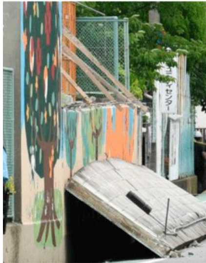
A concrete block wall along a swimming pool, which collapsed during the earthquake (Takatsuki Municipal Juei Elementary School, Osaka Prefecture)
