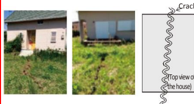
<Examples of housing damage caused by cracks and an image of a crack causing a “completely destroyed” assessment in the 2016 Kumamoto Earthquake>
