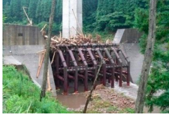
An example of catching driftwood by an erosion control dam of transmission type
