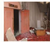
[A hotel damaged by the earthquake]
