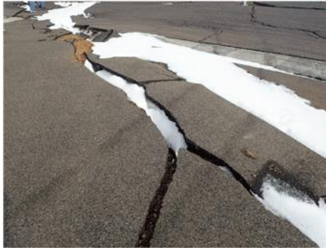
Cracks in the road surface (Nihonmatsu City, Fukushima Prefecture)
