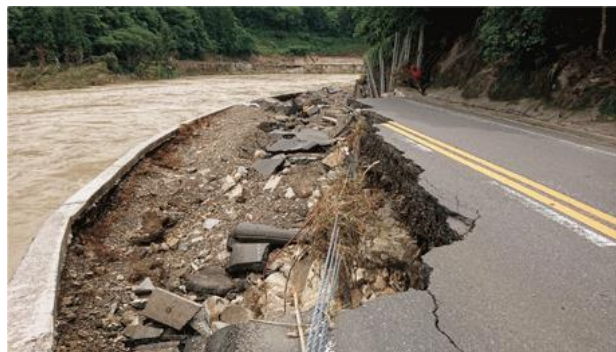
Flooding damage in Kumamoto Prefecture (Kuma Village) (Cabinet Office data)
