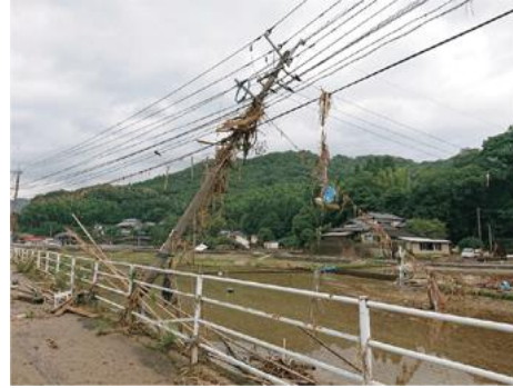
Flooding damage in Kumamoto Prefecture (Kuma Village) (Cabinet Office data)
